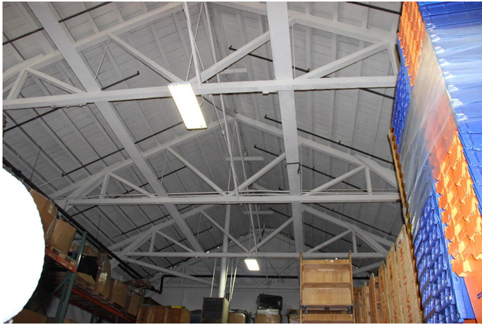
Figure 14. Interior roof framing of warehouse at 1100 17 th Street, looking south, 2014 Source: Christopher VerPlanck
